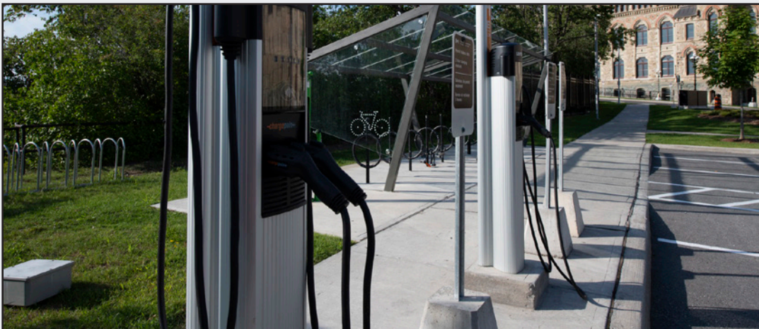
Charging stations for electric vehicles
